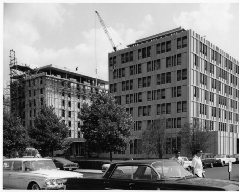
East wing of McCormick Hall under construction in 1966 (image from Cambridge Historical Commission, n.d.).
